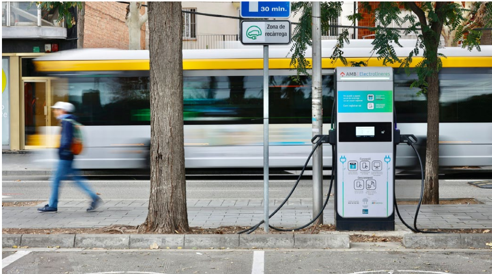
EV charging station
